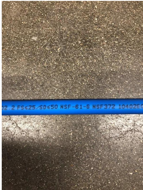
Blue potable PEX line with NSF label
